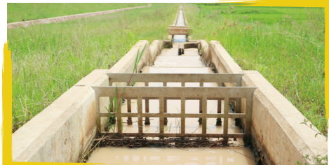
Building Irrigation Management System AGRICULTURE
